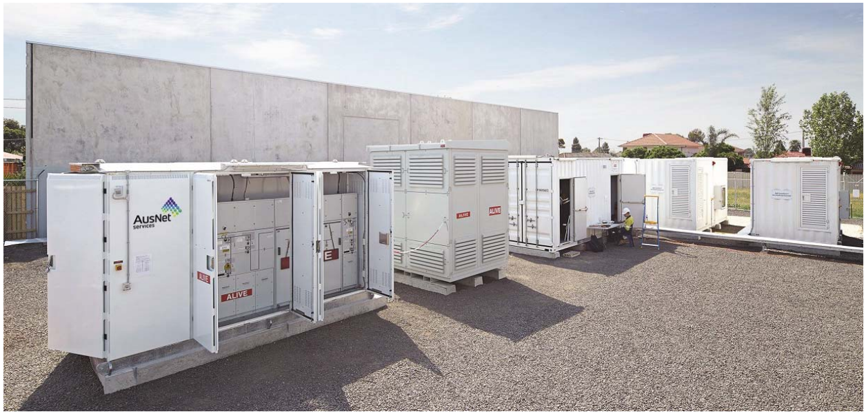
Fig 1: The AusNet Services Grid Energy Storage System, installed in Thomastown (Photo credit: ABB)
